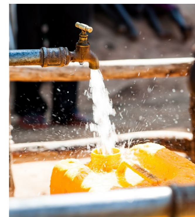
Clean water from a tap connected to a motorized borehole system.
