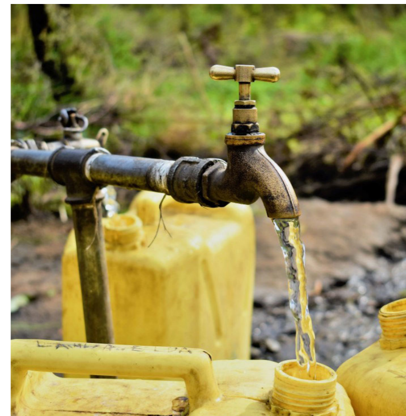
LWF extends clean safe water to persons of concern in Uganda's refugee settlements by drilling and motorising boreholes in the targeted locations.
