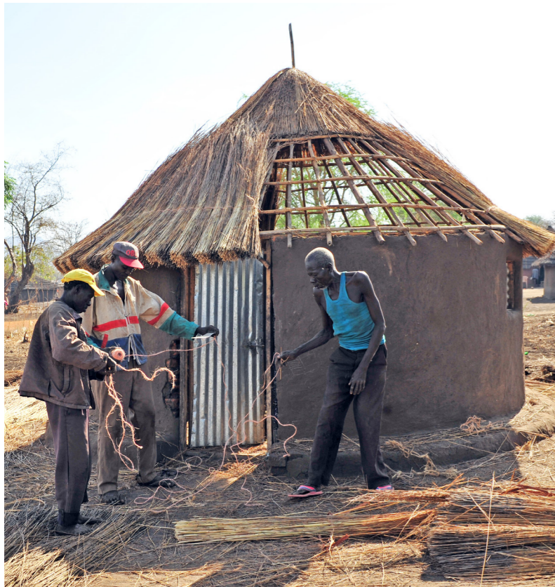
LWF extends Shelter services and Construction materials to persons of concern in Uganda's refugee settlements.
